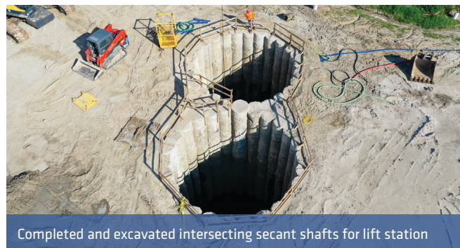
Schnabel's jet grout system used for large-diameter soil mixing on the project
